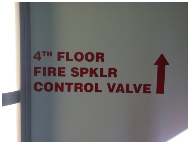
Photo 3 – Floor Control Valve Identification
