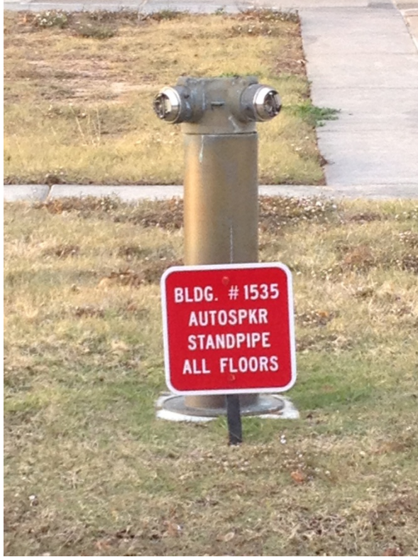
Photo 4 – Remote Standpipe/Sprinkler Identification
